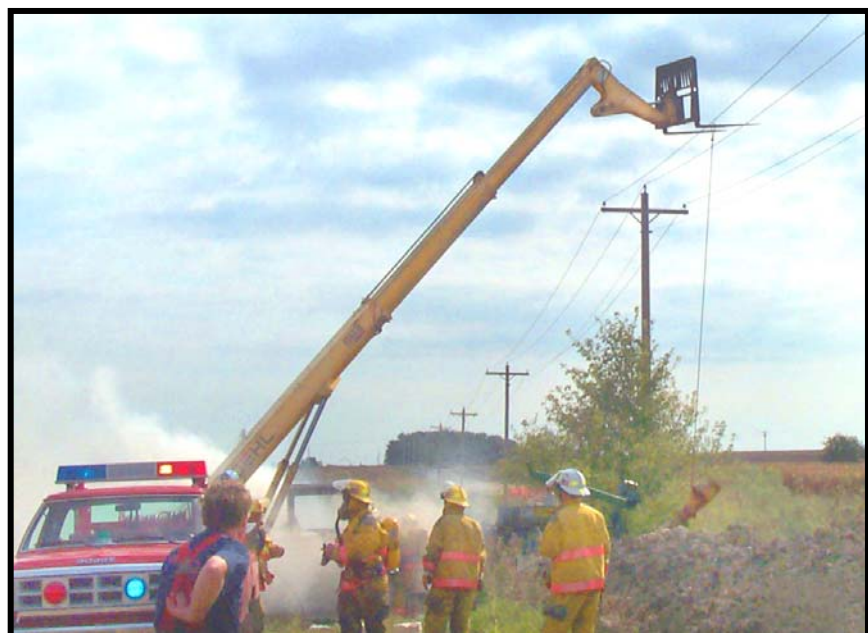
Photo 1 – View of firefighters at the scene, showing the forklift near the powerlines and the pump suspended by a wire rope cable.
