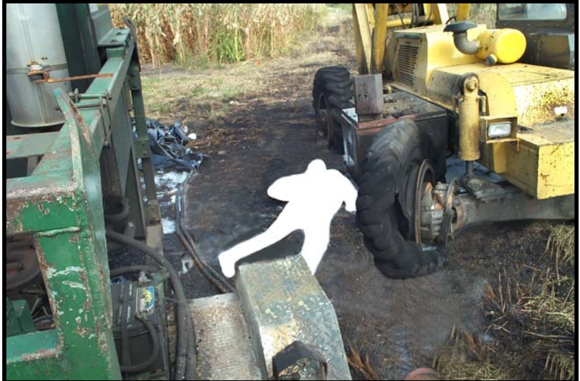
Photo 3 – View between the forklift and the hydraulic power unit, facing north, showing position of the victim after he fell to the ground.
