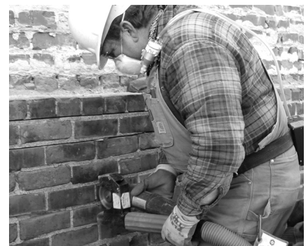
Something missing? Tuckpointing minus the cloud of dust—thanks to modifications developed and tested by OEH scientists.
